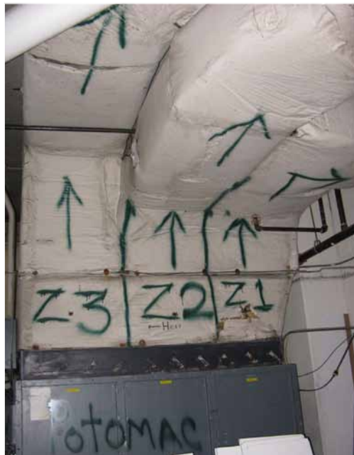
Auditors inventory and measure equipment efficiency.
