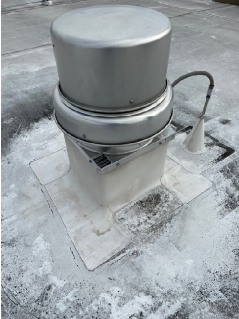
Figure A: Rooftop Exhaust Fan (Greenheck GB)
