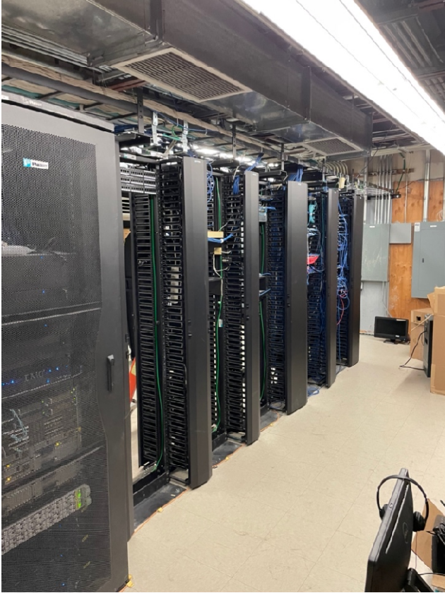
Figure E: Server Room
