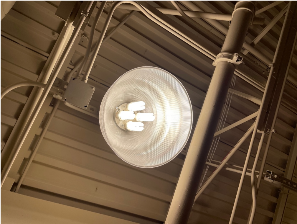
Figure F: Primary Sales Floor Lighting
