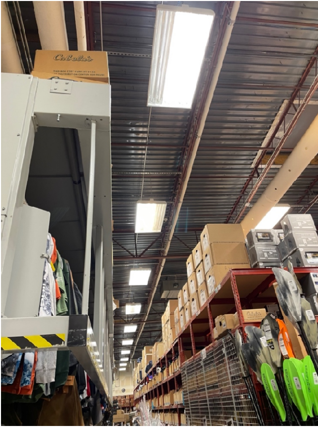
Figure G: Warehouse Highbay Lighting
