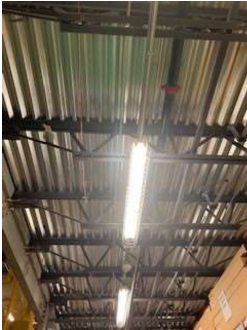
Figure D: Warehouse Track Lighting
