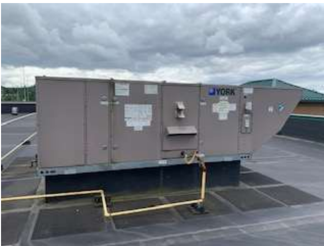
Figure B: RTU (YORK)
