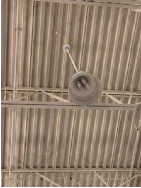
Figure C: Primary Sales Floor Lighting
