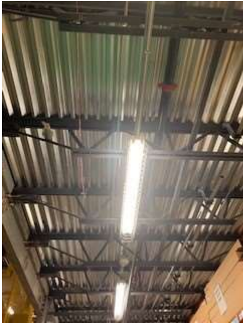
Figure D: Warehouse Track Lighting
