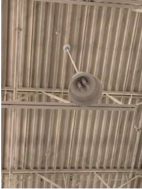
Figure C: Primary Sales Floor Lighting
