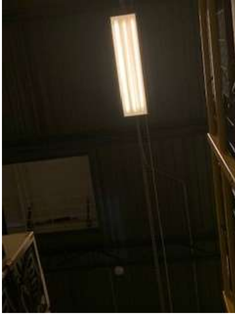
Figure E: Warehouse Lighting, 3 Lamp
