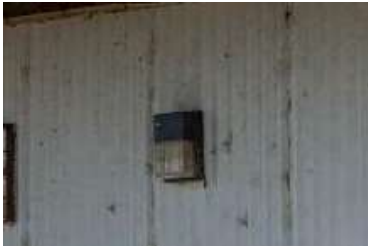
Figure K: Existing Fixture N
