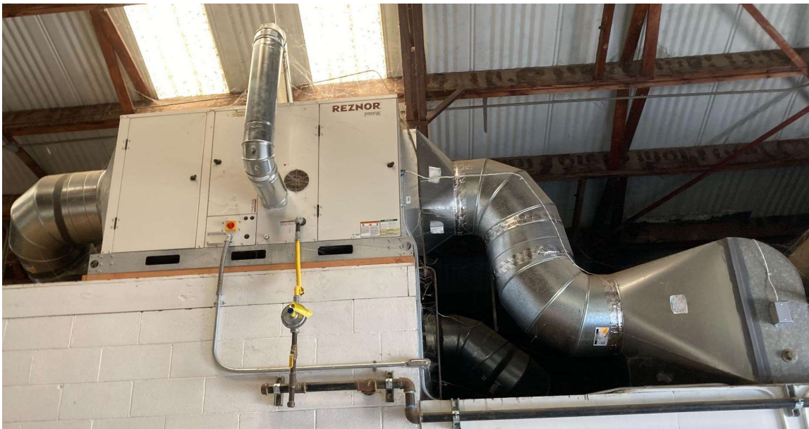
Figure T: Reznor Gas Fired Dryer
