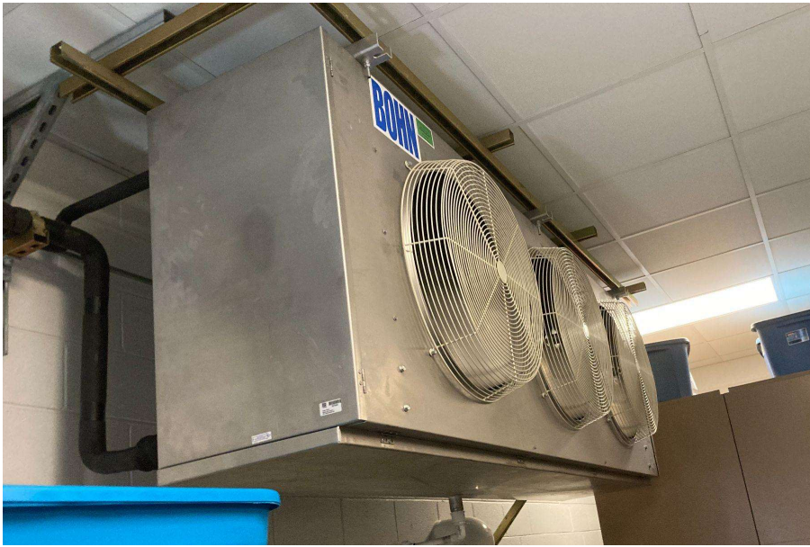
Figure S: Indoor Evaporator of Walk-In Cooler
