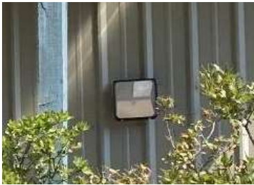
Figure L: Existing Fixture O
