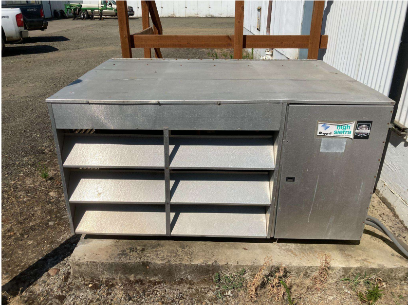
Figure R: Outdoor Condensing Unit
