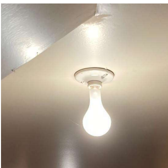
Figure C: Existing Fixture E
