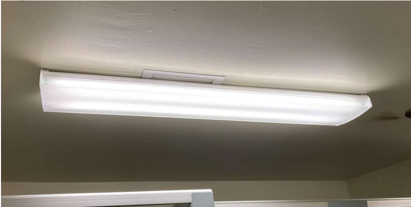
Figure A: Existing Fixture A
