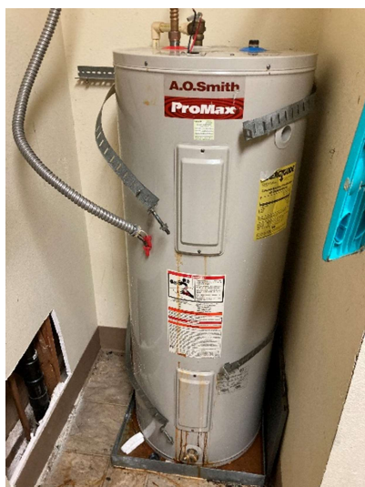
Figure E Electric Storage Tank Domestic Water Heater
