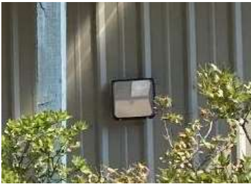
Figure L: Existing Fixture O
