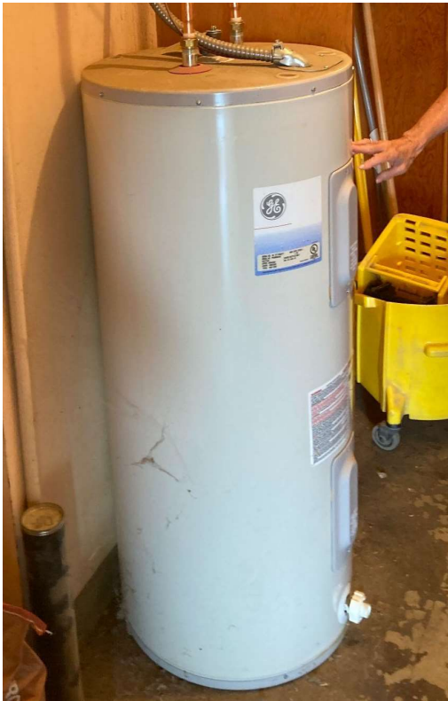
Figure V: Typical Domestic Water Heater
