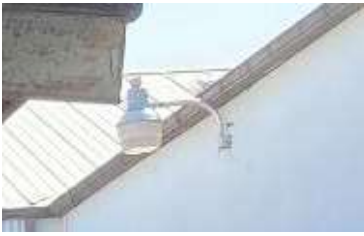
Figure J: Existing Fixture M
