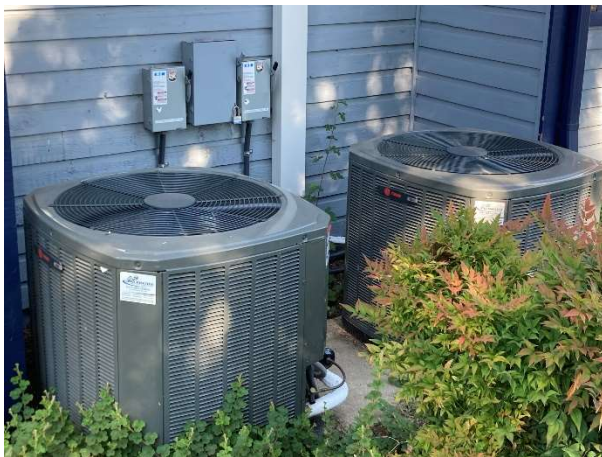
Figure D: Typical Split System Heat Pump Outdoor Units
