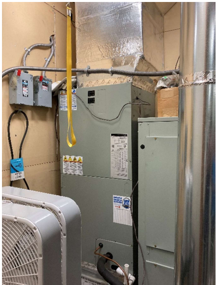
Figure B: Typical Split System Heat Pump Indoor Unit (Lower Level Mechanical Room)
