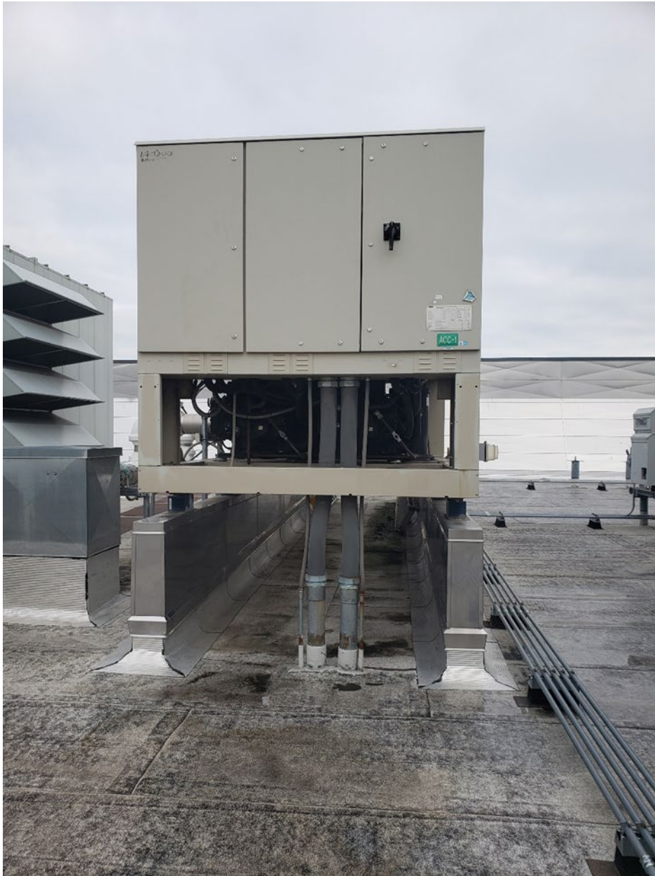
Figure E : Roof Mounted Air Cooled Chiller (ACC-1)
