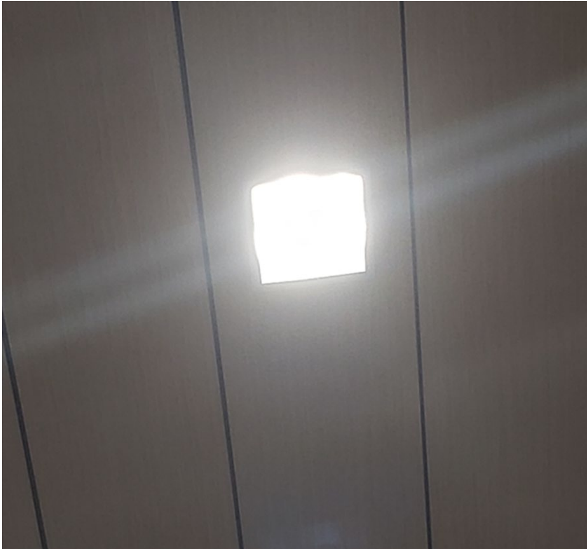
Figure A: Primary Lobby Lighting
