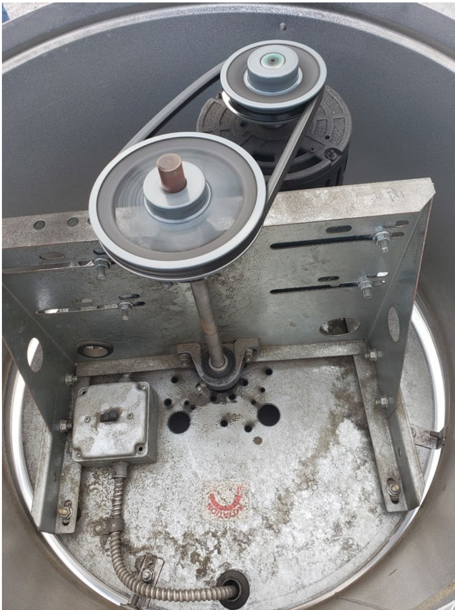
Figure G: Roof Mounted General Restroom Exhaust Fan (EF-1)
