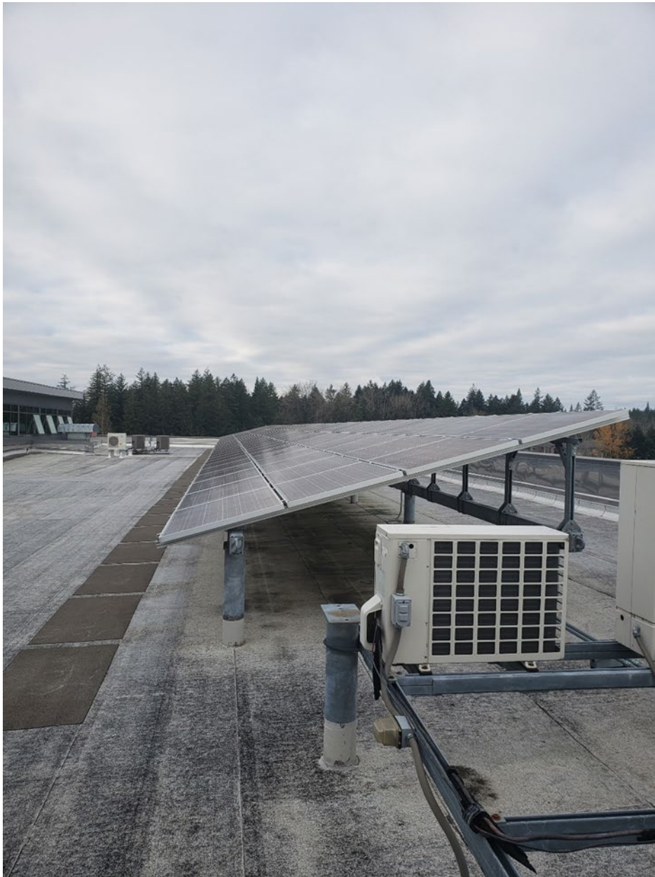
Figure F: Roof Mounted PV Solar Array
