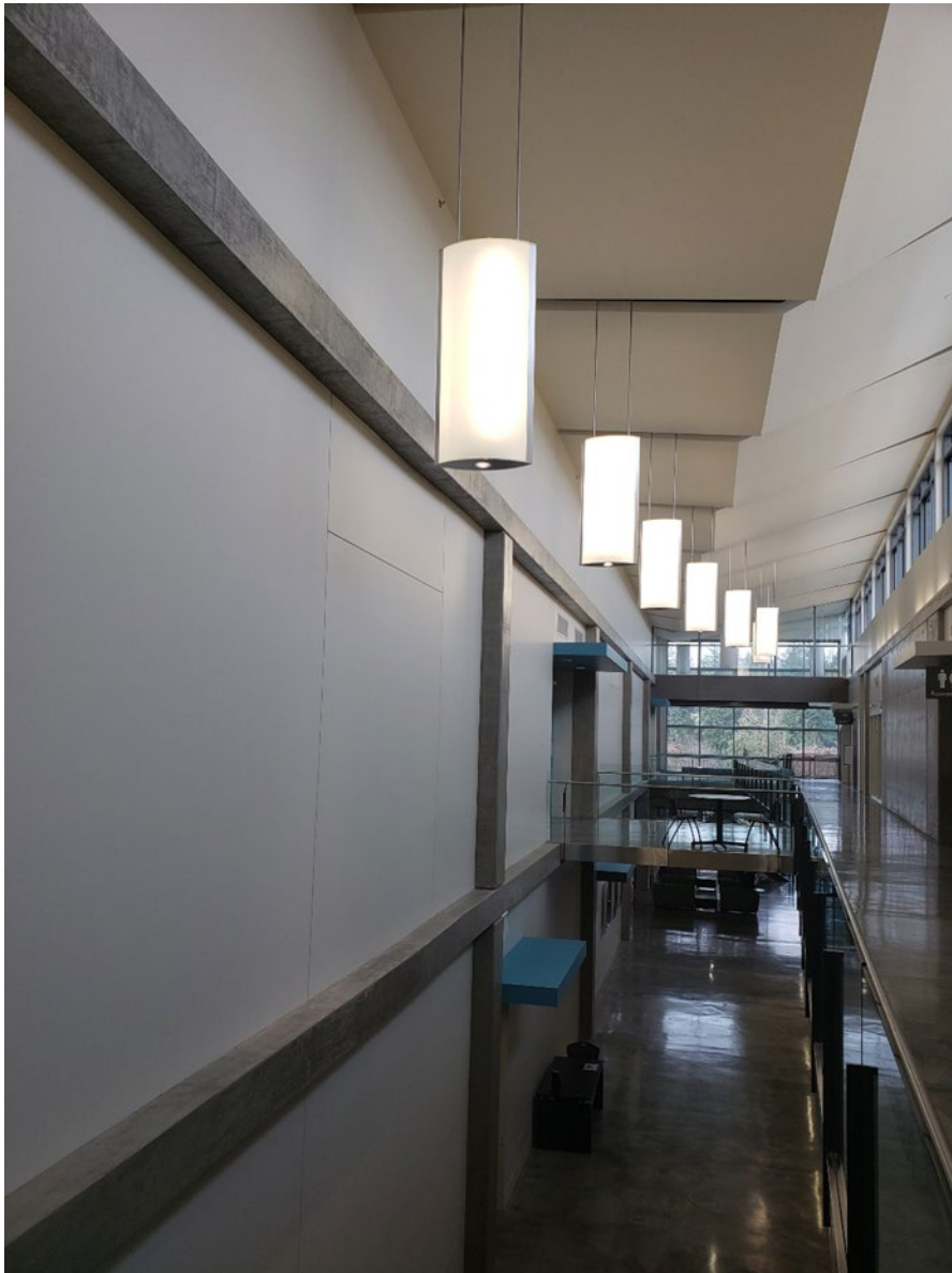
Figure B: Pendant Hung Fixtures in Corridor
