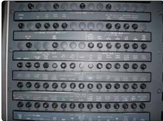
Figure 9-173. Circuit breaker panel.
