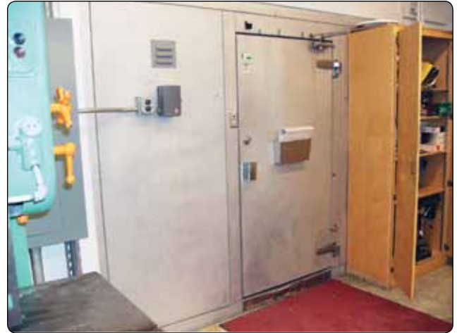
Figure 7-44. Walk-in freezer for storing prepreg materials.
