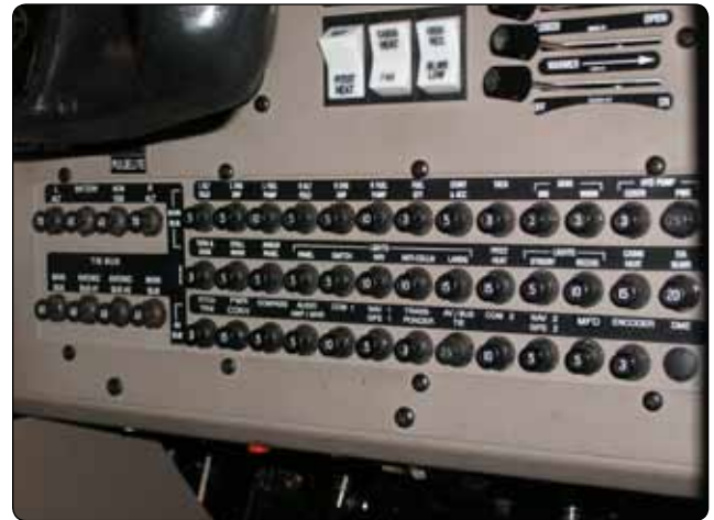
Figure 9-83. Light aircraft circuit breaker panel.
