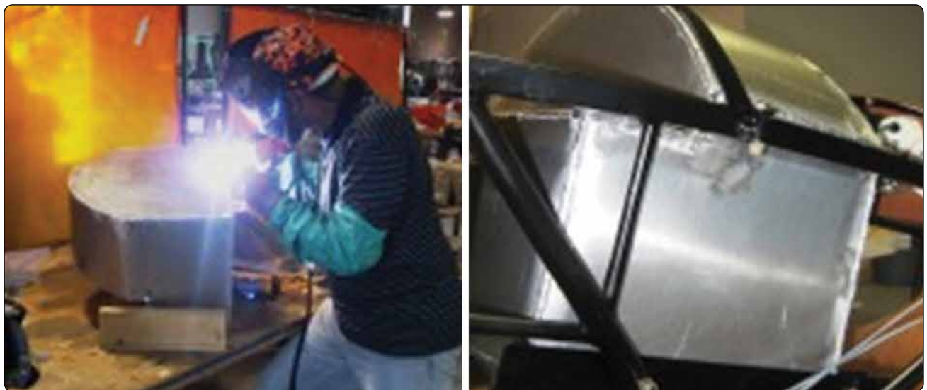
Figure 14-91. A rigid removable fuel tank with welded seams is repaired by welding.
