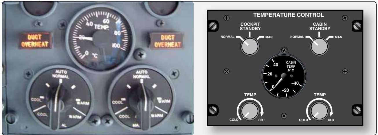
Figure 16-70. Typical temperature selectors on a transport category aircraft temperature control panel in the cockpit (left) and a business jet (right). On large aircraft, temperature selectors may be located on control panels located in a particular cabin air distribution zone.
