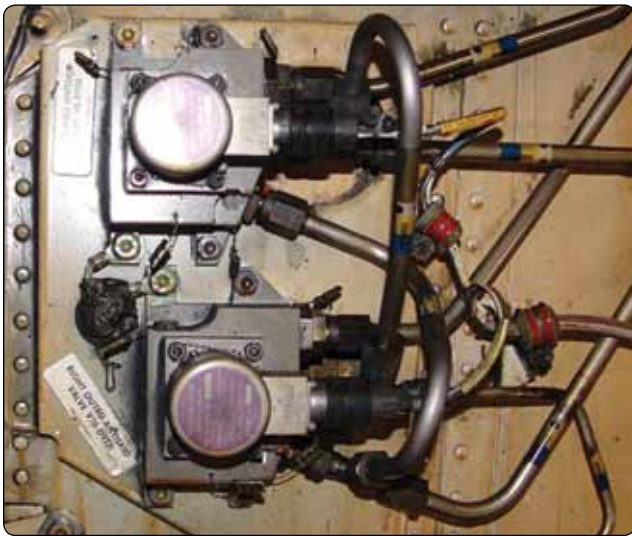
Figure 13-111. Two antiskid control valves with associated plumbing and wiring.
