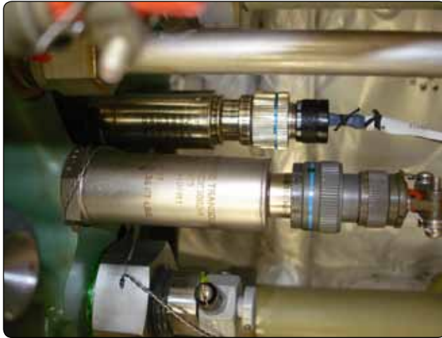
Figure 12-11. Temperature and quantity sensors.
