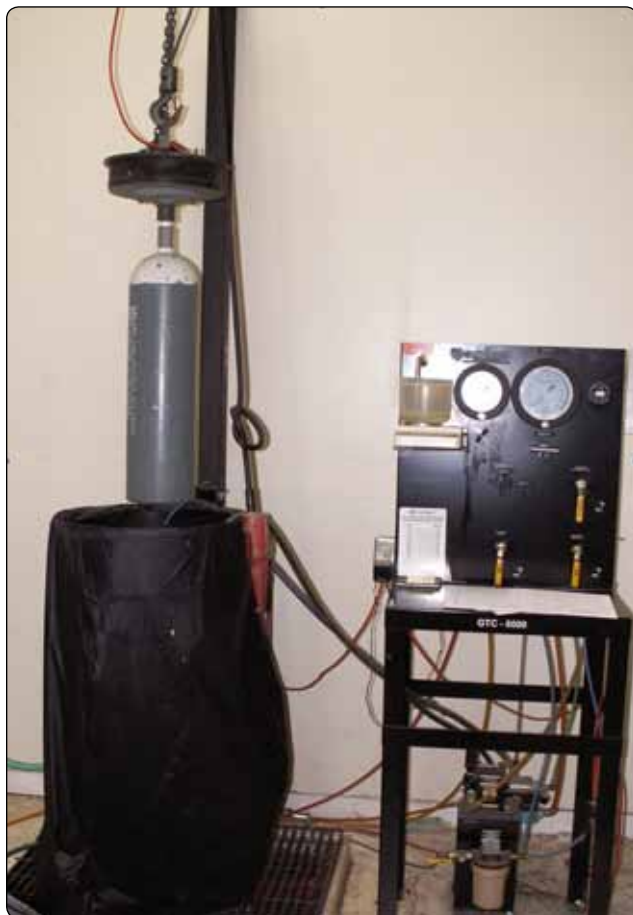
Figure 16-9. This test stand is used for hydrostatic testing of oxygen cylinders. The water-filled cylinder is lowered into the barrel on the left where it is pressurized to the proper level as monitored via gauges mounted on the control panel. A displacement container on the top left of the control board collects water from the barrel to measure the expansion of the cylinder when pressurized to ensure it is within limits.
